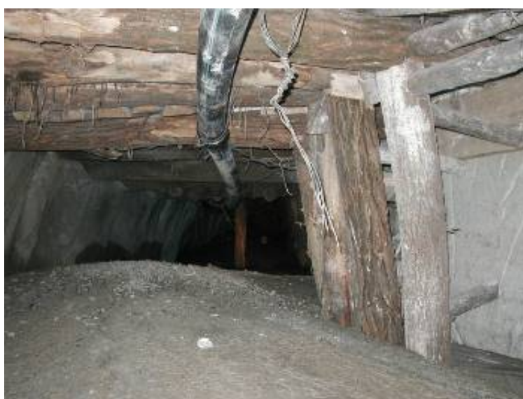
Fig. 10. The mixture is transported through the steel piping.
