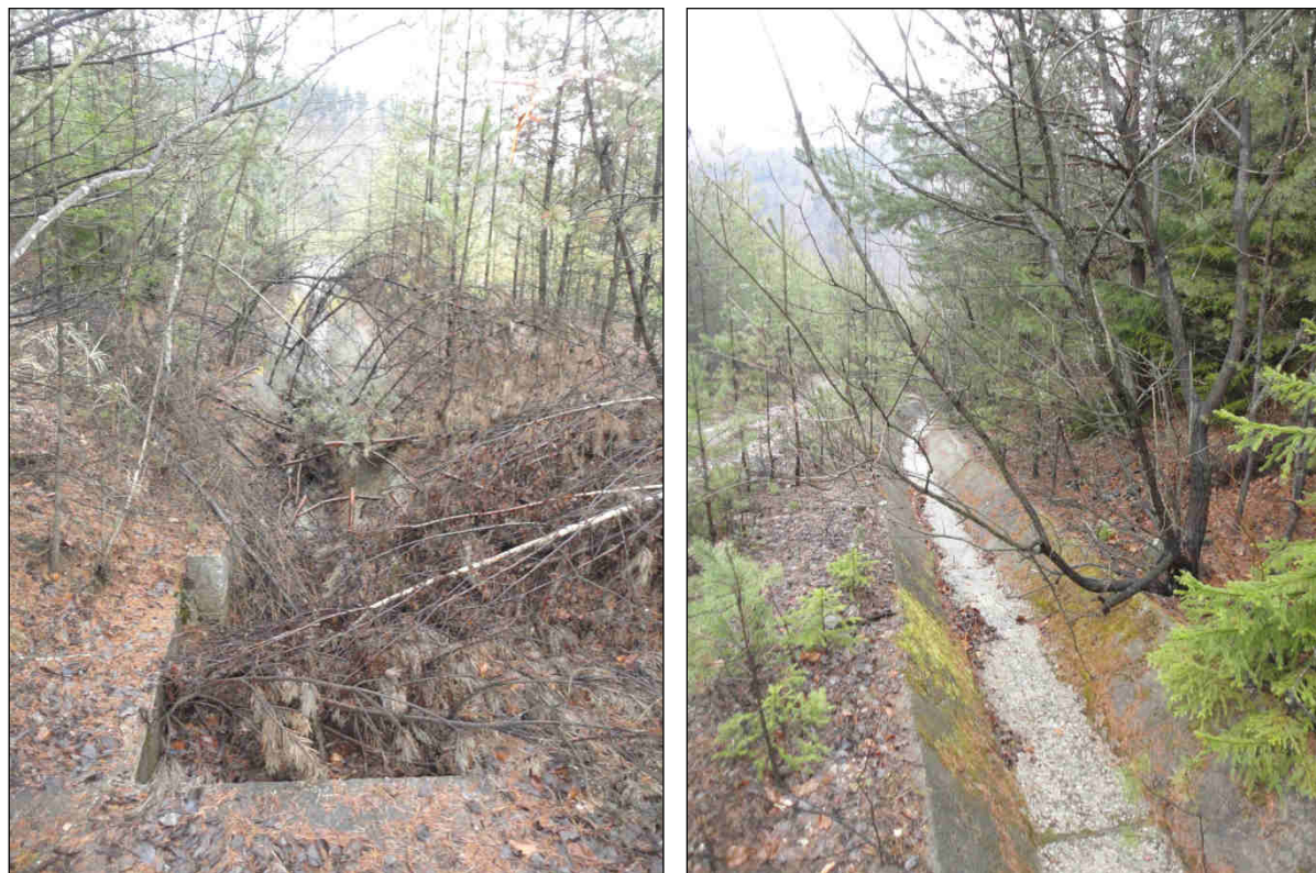
Fig. 8. 9 Concrete channels are in the bad condition in some parts (photo: authors).
