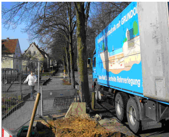
Fig. 3. Old cable replacement project in Uelzen. The cable path is situated beneath the alley of trees.
