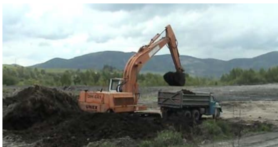
Fig. 3. Machines in operation on the Central Heap [1].
