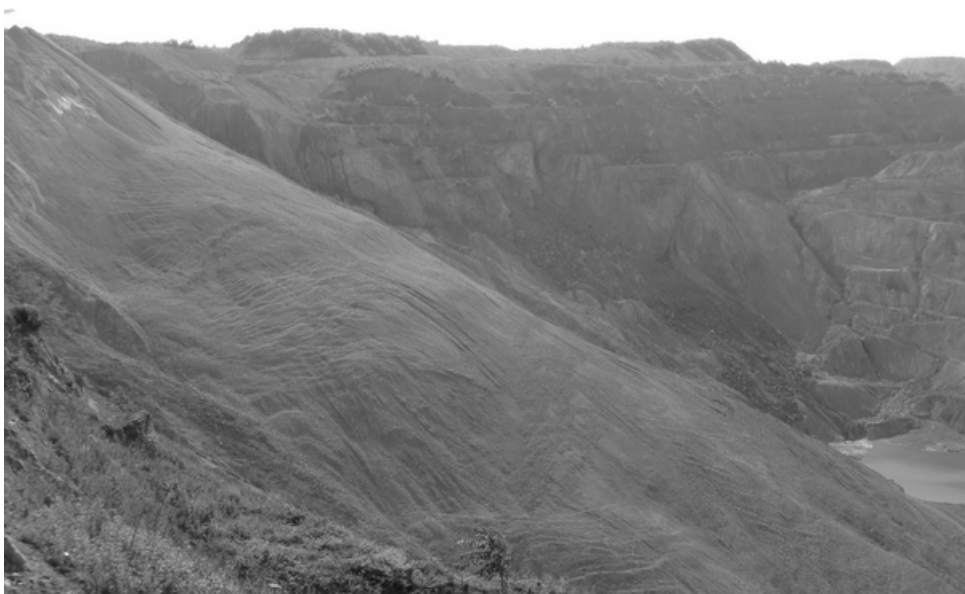
Fig. 9. View of the slope with noticeable swelling.
