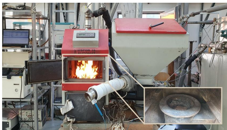
Fig. 2. Small pellet boiler with retort burner.
